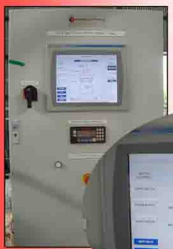
Control Panels can be manufactured to meet our clients specific requirements, control upstream equipment and incorporate touch screen or SCADA.
